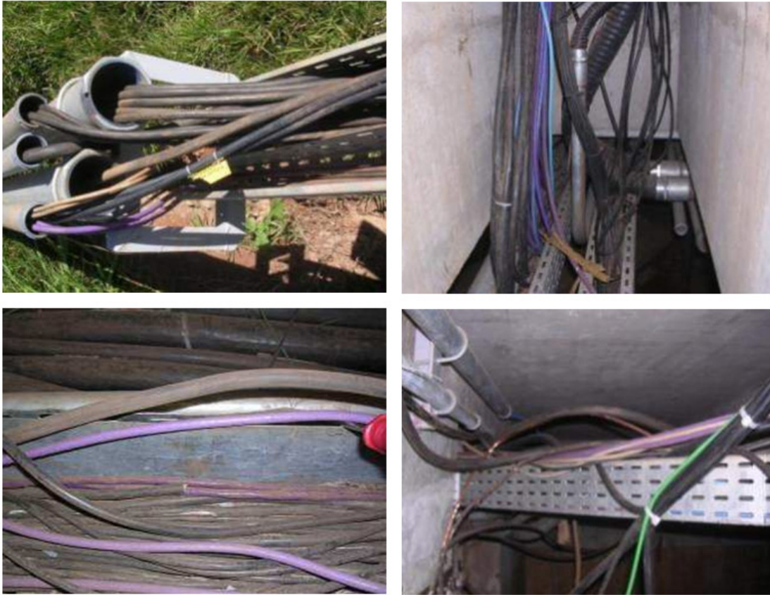
Figure 22 d – Example of Profibus Cables near the power source cable
